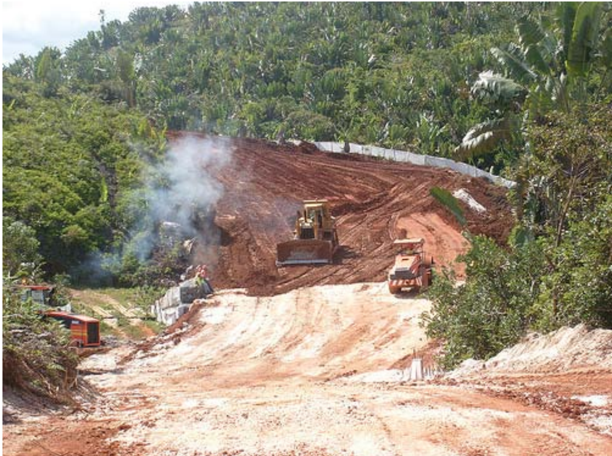
Land construction in Madagascar. Photo by Foko Madagascar, used with author's permission.
